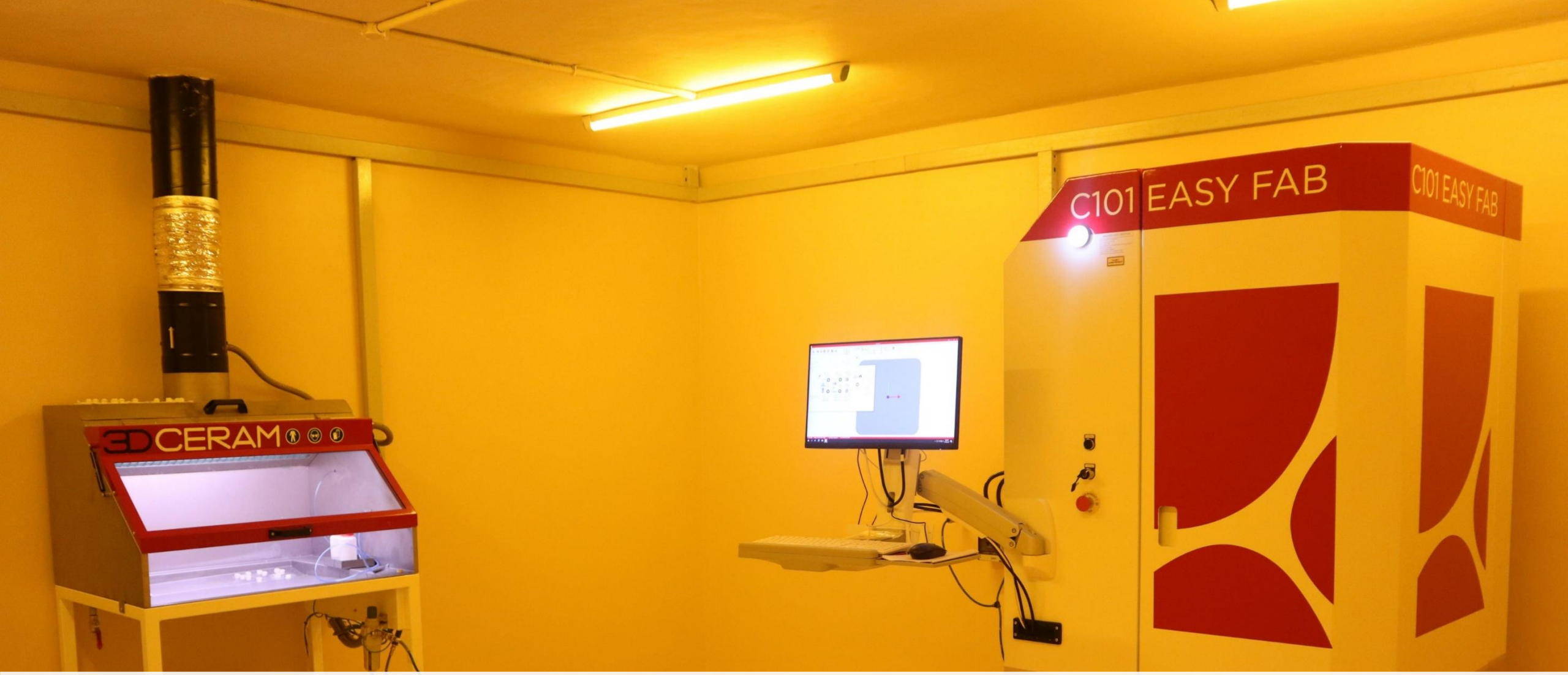
Ceramic 3D Printer installed and commissioned at Industrial Ceramics, Hosur
